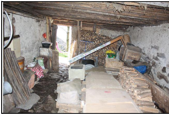
Locale PT / Erdgeschoss
