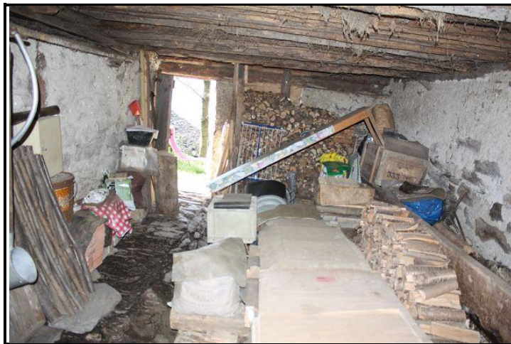
Locale PT / Erdgeschoss
