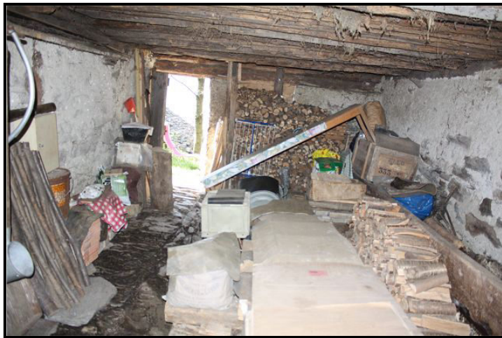
Locale PT / Erdgeschoss
